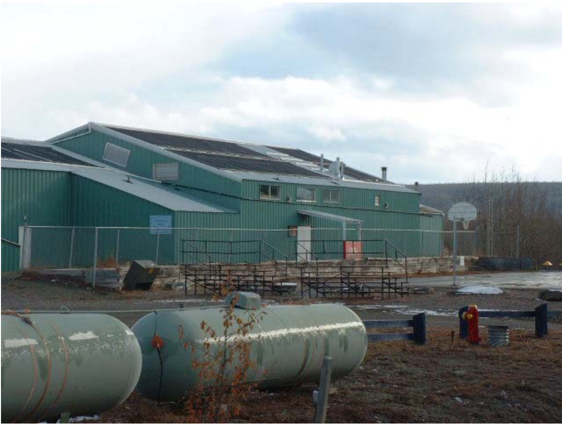
Arena Propane Tanks
