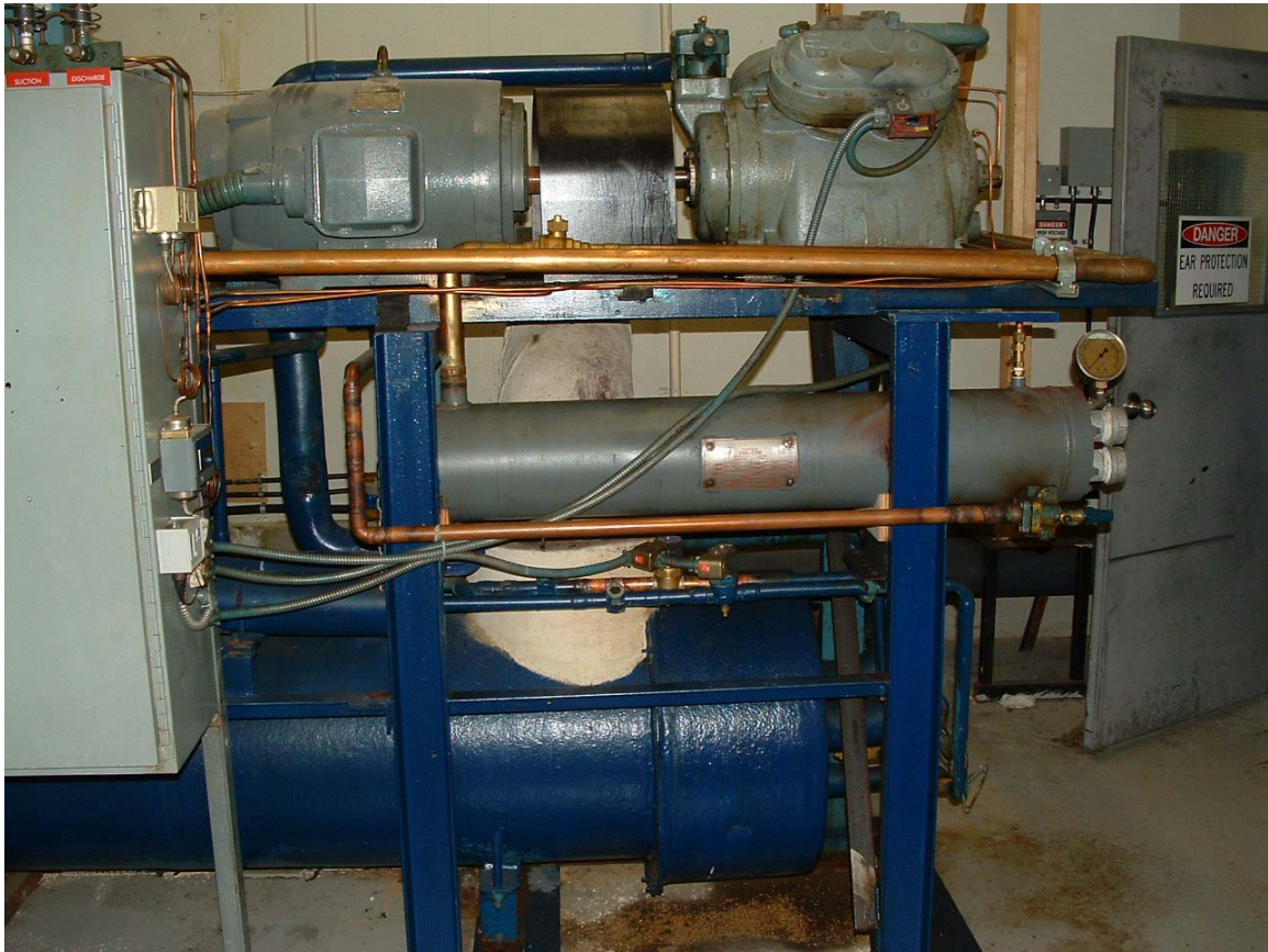
Arena Ice Plant
