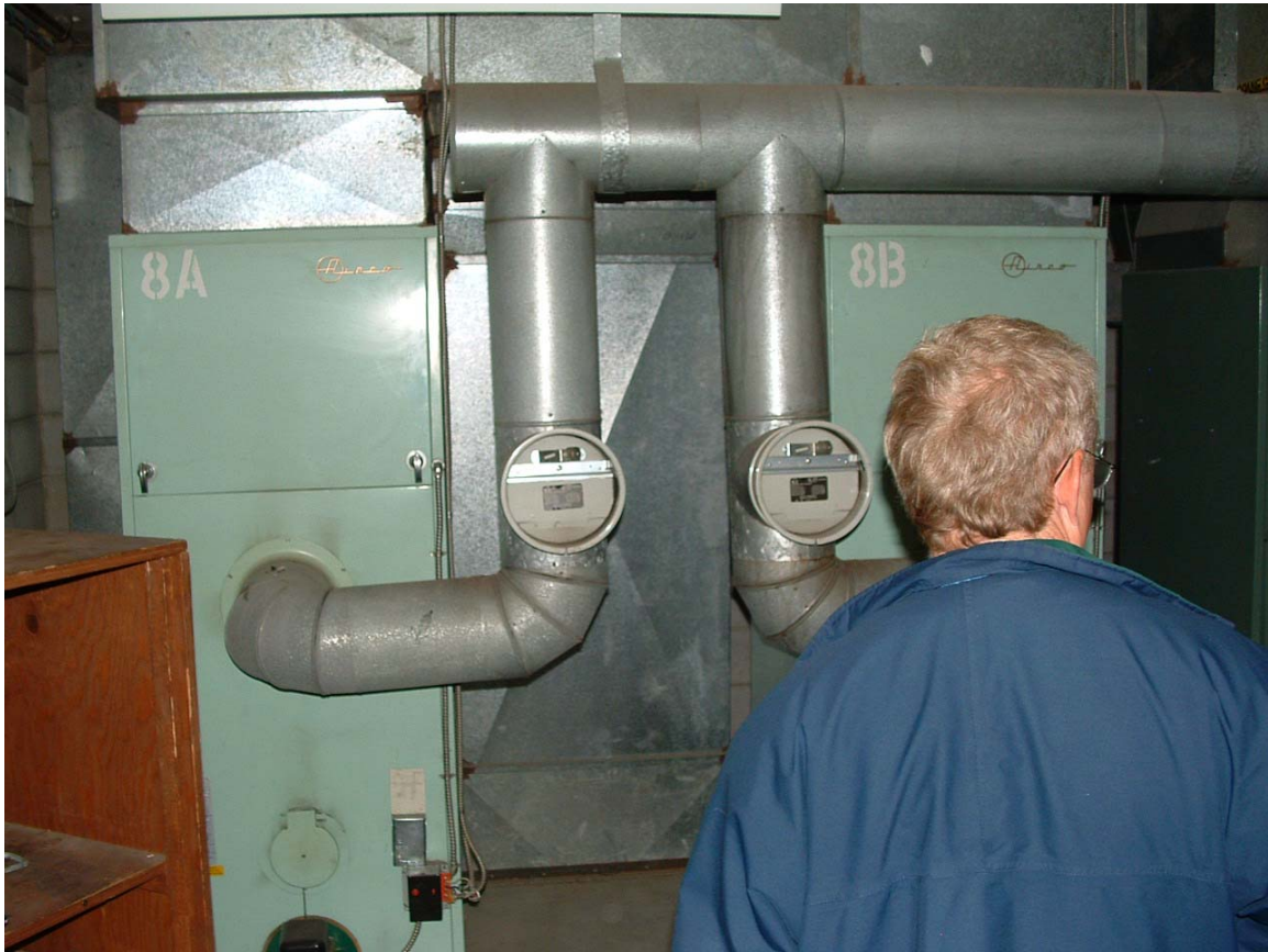
Arena Mechanical Room
