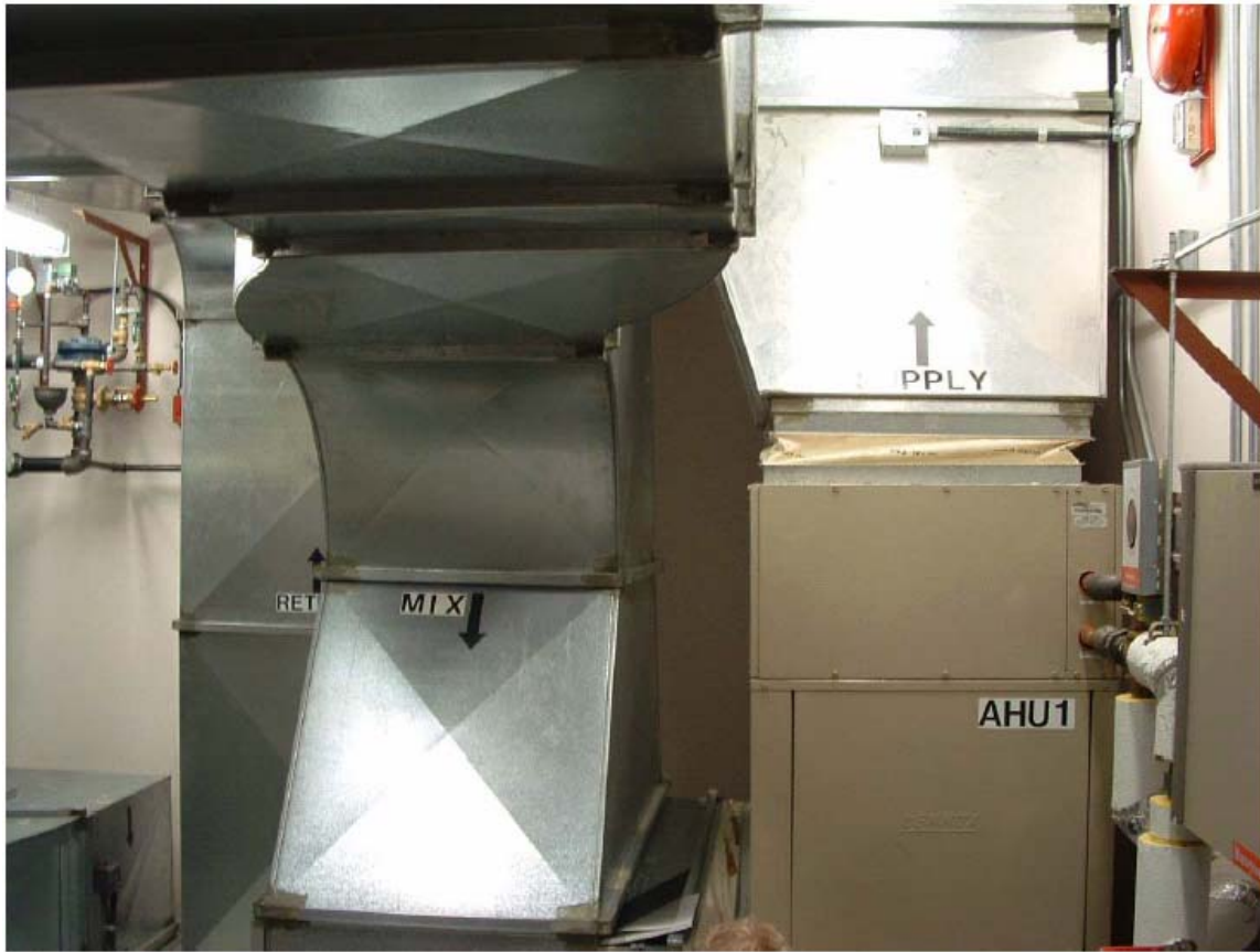
Convention Centre Mechanical Room
