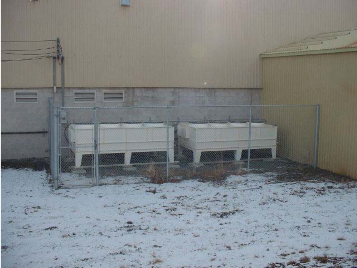
Arena Cooling Towers
