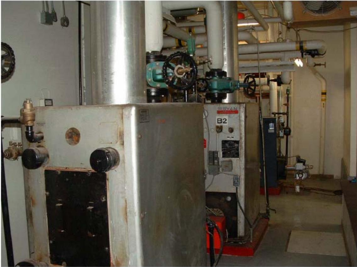
School Mechanical Room
