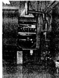
Figure 12 - Community Hall, Domestic Hot Water Heater and Decommissioned Gas Fired Furnace
