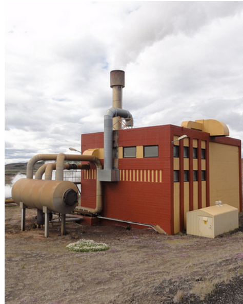
3 MW power and heating plant in northern Iceland, source: ThinkGeoENERGY
