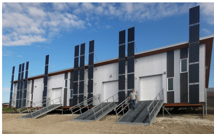
12.1 kW solar array on the Old Crow research facility, source: kobayashi + zedda architects
