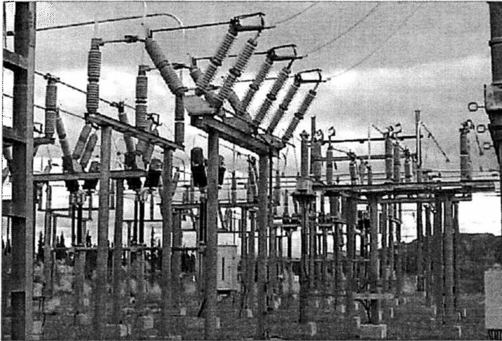
Takhini substation belonging to Yukon Energy Corporation.
