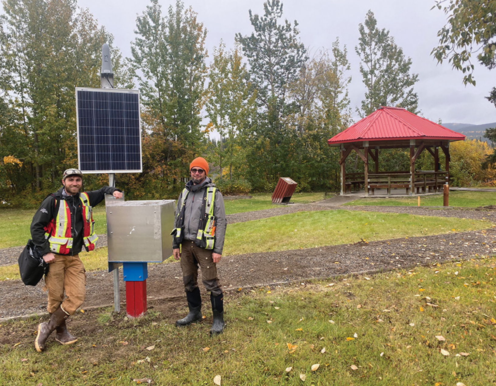
Groundwater Technologists Norbert Botca (right) and Cole Fischer (left) pictured after the installation of a telemetry system on a monitoring well at the Carmacks playground (Brendan Mulligan, 2023).
