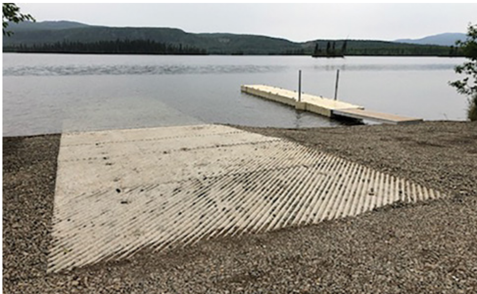
A new dock and boat launch was installed at Twin Lakes Campground.
