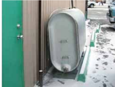
Vehicle bumpers could contact this unprotected tank. It is likely leaning due to a bumper having pressed against it.
