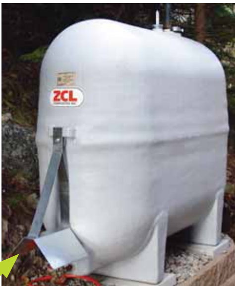
Fiberglass single-wall home-heating oil tank. Note the protective shield over the fuel outlet valve and piping.
