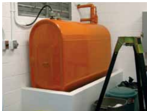
An indoor tank with secondary containment. Notice the fill and vent pipes terminate outdoors.
