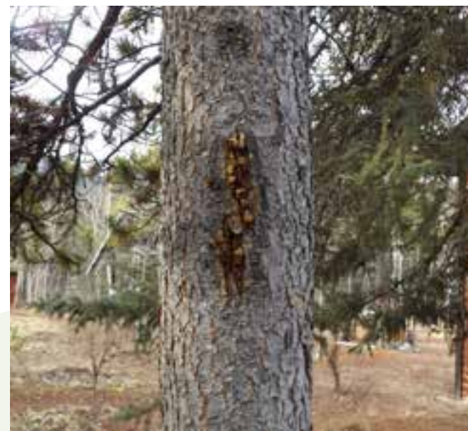
PHOTO 50 Old bear damage or mechanical damage from axe cuts, Annie Lake road.
