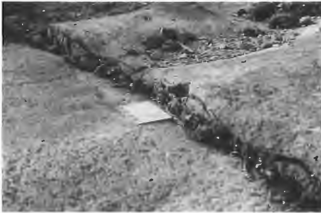
Figure 7. Neotectonic fault at Cheam View (Location 2).
