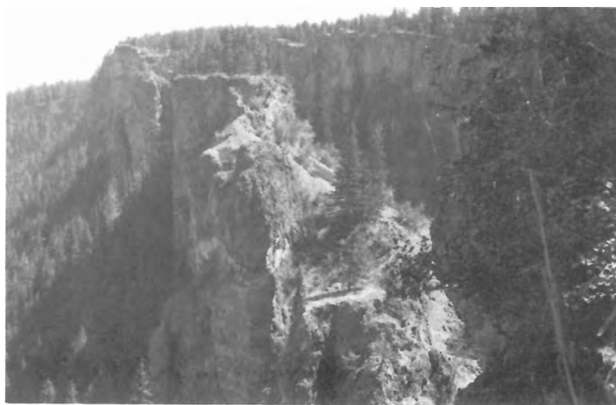
Figure 10. Tension cracking and separation at the top of Shell Creek slide scarp.
