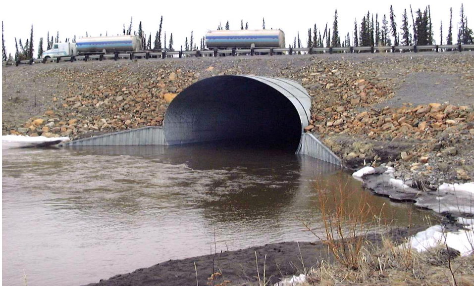
Snag Creek Multiplate, showing headwall, Feature BC167
