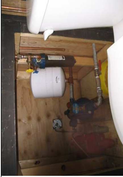
Photo 190: 5636 Jet pump and pressure tank.
