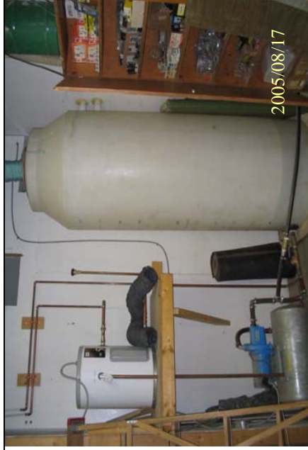
Photo 191: 5640 Water tank and jet pump.
