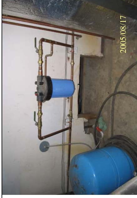
Photo 194: 5650 Water system. (pressure tank and filter)
