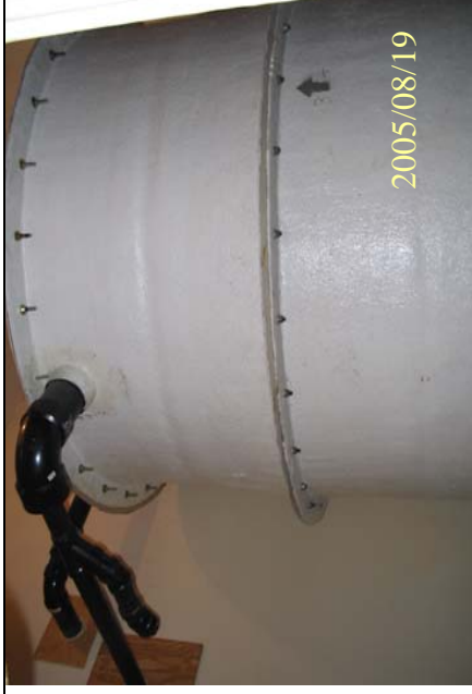
Photo 225: 2575 Water storage tank.
