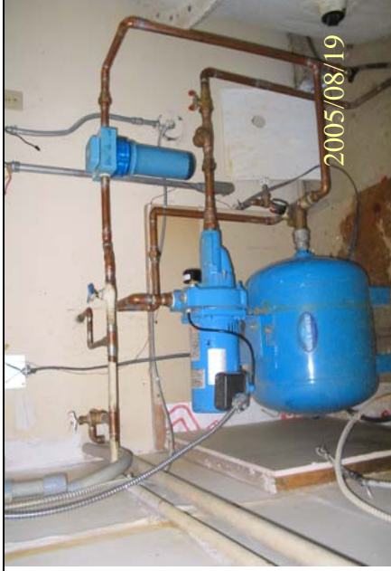
Photo 223: 2575 Jet pump, pump controls and inline filter.
