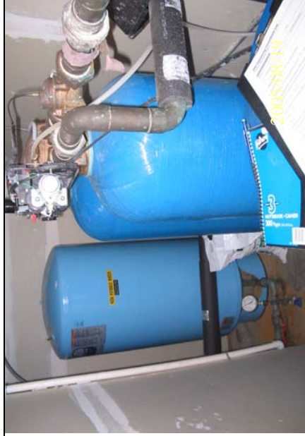
Photo 230: 2599 Pressure tank, pump controls and softener system.
