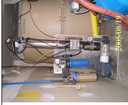
Photo 234: 2599 Reverse osmosis system (front) water storage tank (back)
