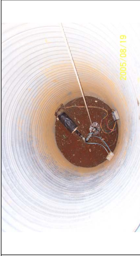
Photo 086: 2599 Wellhead in pit.
