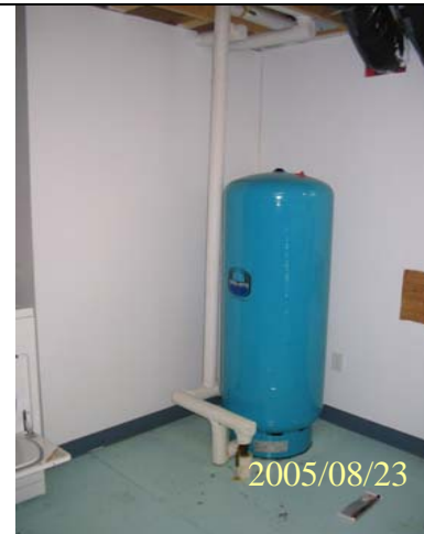
Photo 200: M0227 Pressure tank.
