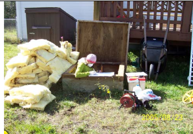
Photo 386: M0026 Well enclosure.
