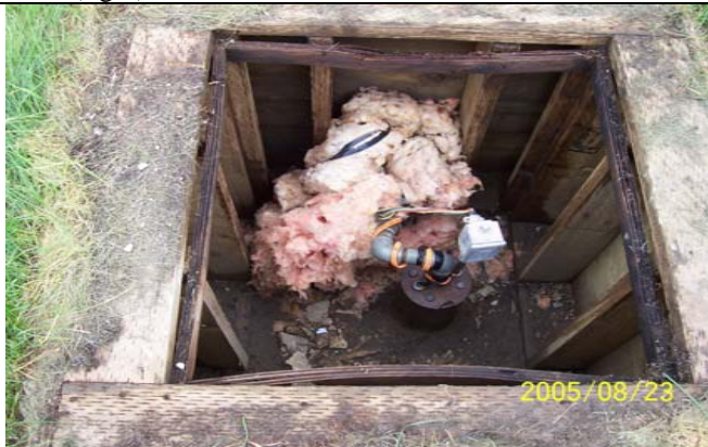
Photo 379: M0156/M0226 Well enclosure and wellhead.
