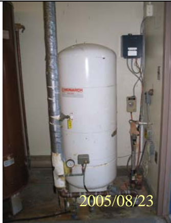
Photo 208: 5672 Water system. (pump controls, pressure tank)
