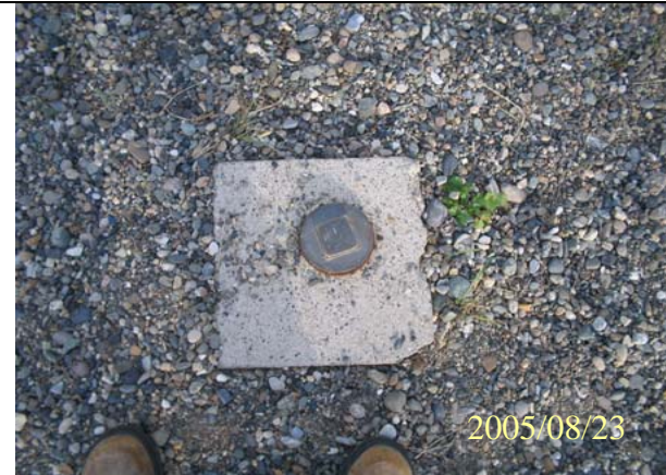
Photo 214: 5672 Potential septic clean out?
