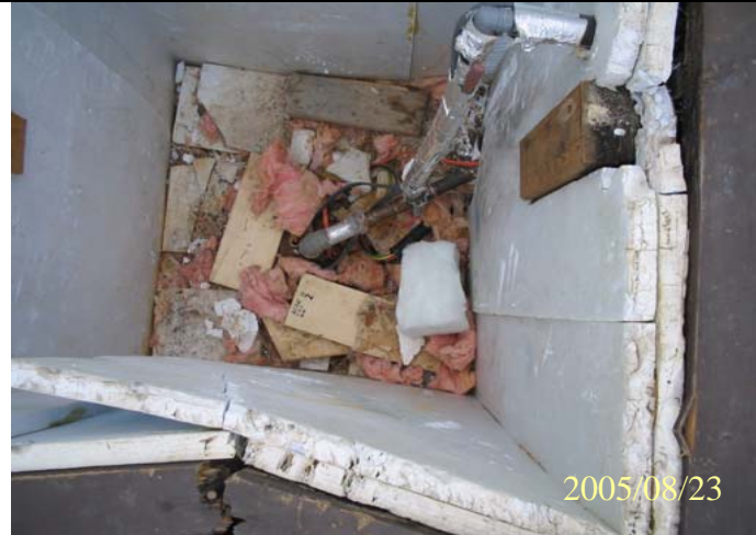
Photo 209: 5672 Well enclosure and wellhead.
