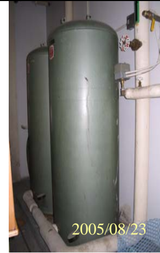
Photo 204: 5676 Water System. (pump controls and pressure tanks)
