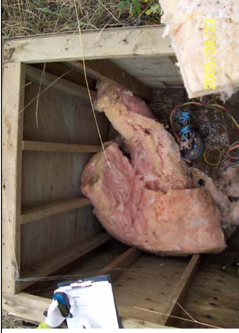
Photo 402: 5678 Well enclosure and wellhead.
