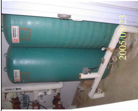
Photo 202: Water system. (pressure tanks & pump controls)
