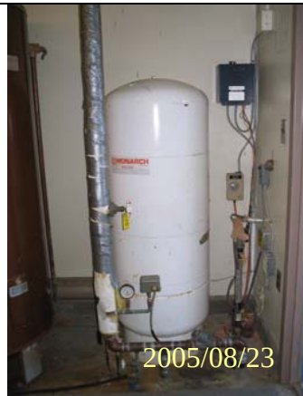
Photo 208: 5672 Water system. (pump controls, pressure tank)
