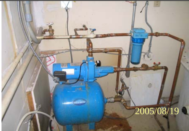
Photo 223: 2575 Jet pump, pump controls and inline filter.
