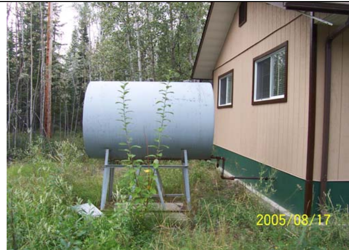
Photo 057: 5650 On site AST.
