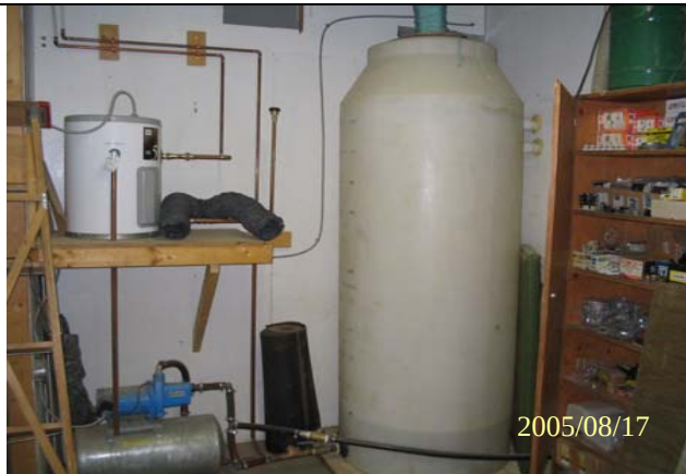
Photo 191: 5640 Water tank and jet pump.
