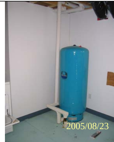
Photo 200: M0227 Pressure tank.
