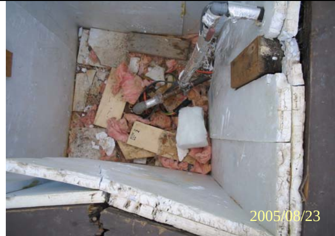
Photo 209: 5672 Well enclosure and wellhead.
