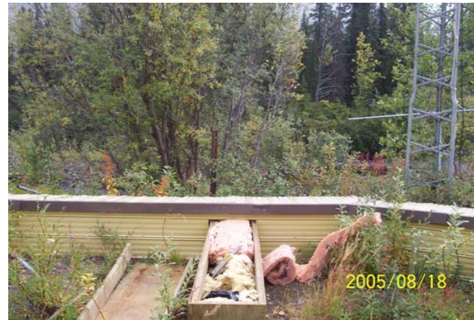
Photo 067: 2600 Wellhead with surrounding enclosure and utilidor.
