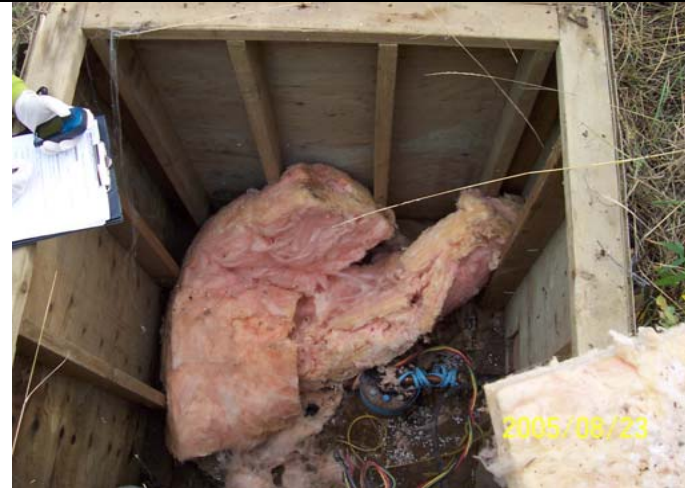
Photo 402: 5678 Well enclosure and wellhead.
