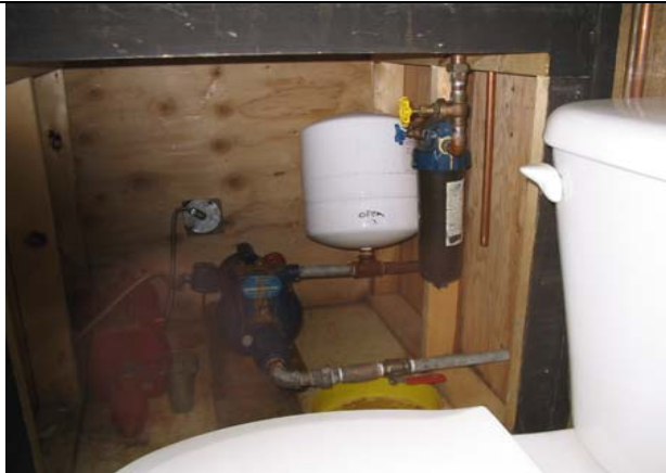
Photo 190: 5636 Jet pump and pressure tank.
