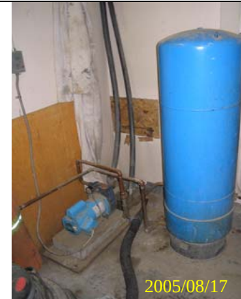
Photo 192: 5629 Grader station pressure tank and jet pump.
