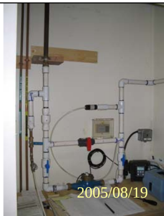
Photo 236: 2592 Chlorination system, flow meter, and associated plumbing.
