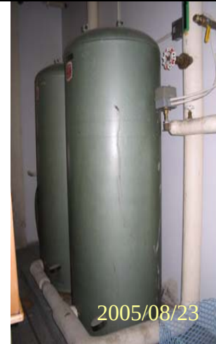
Photo 204: 5676 Water System. (pump controls and pressure tanks)
