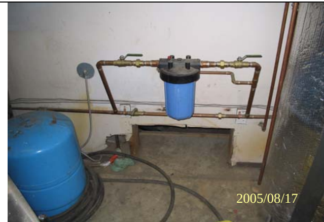
Photo 194: 5650 Water system. (pressure tank and filter)
