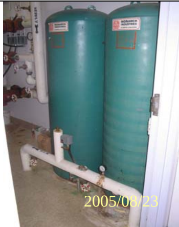
Photo 202: Water system. (pressure tanks & pump controls)
