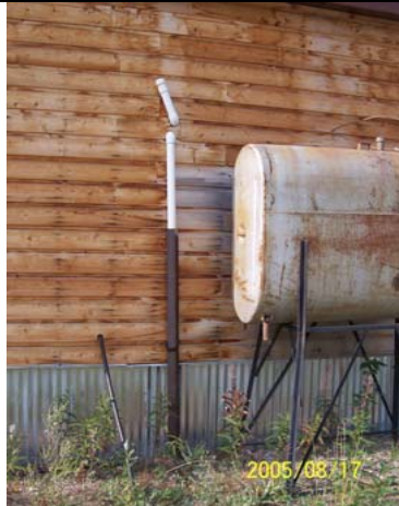
Photo 037: 5640 Water fill and AST.
