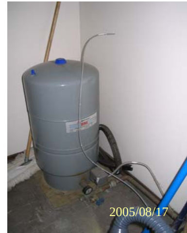
Photo 0189: 5653 Pressure tank and pump controls.
