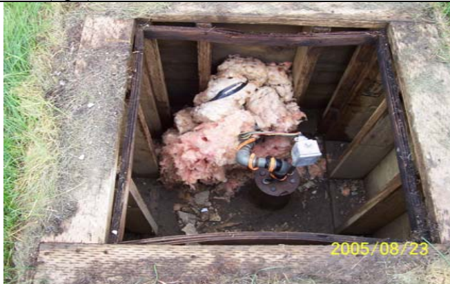
Photo 379: M0156/M0226 Well enclosure and wellhead.
