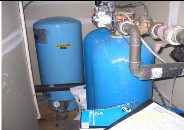
Photo 230: 2599 Pressure tank, pump controls and softener system.
