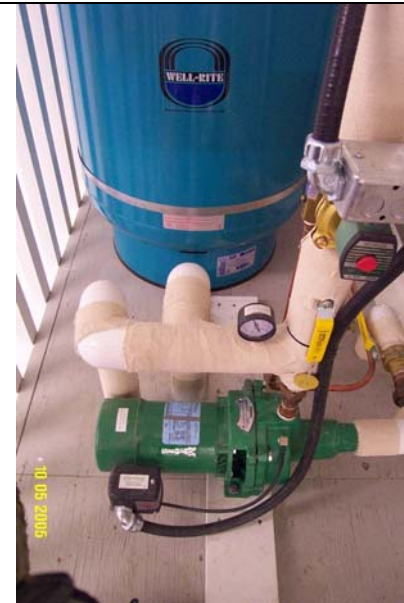
Photo 0098: 1421 Pressure Tank and System
