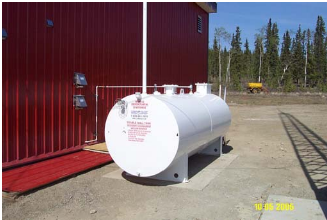
Photo 0093: 1421 Above Ground Storage Tank
