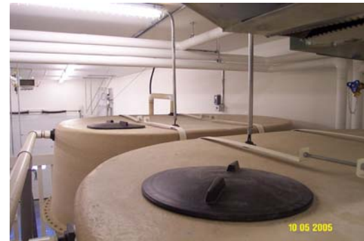
Photo 0097: 1421 Water Storage Tanks (in firehall)
