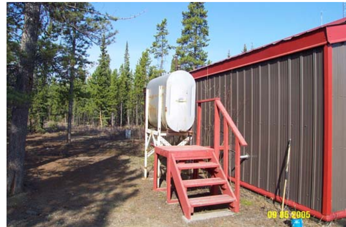
Photo 0077: Above Ground Fuel Storage Tank
