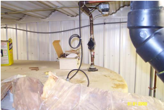
Photo 0107: 1950 Solenoid and Water Storage Tank
