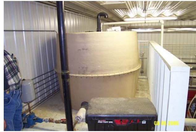
Photo 0066: 1953 Firehall 1250gal Water Storage Tank
