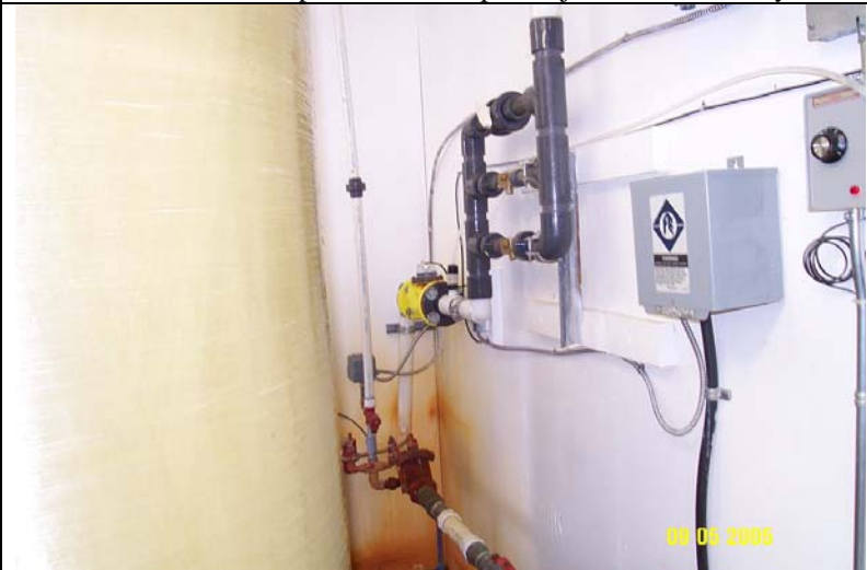
Photo 0070: 1953 Pumphouse Iron Duplex Injection Chlorine System
