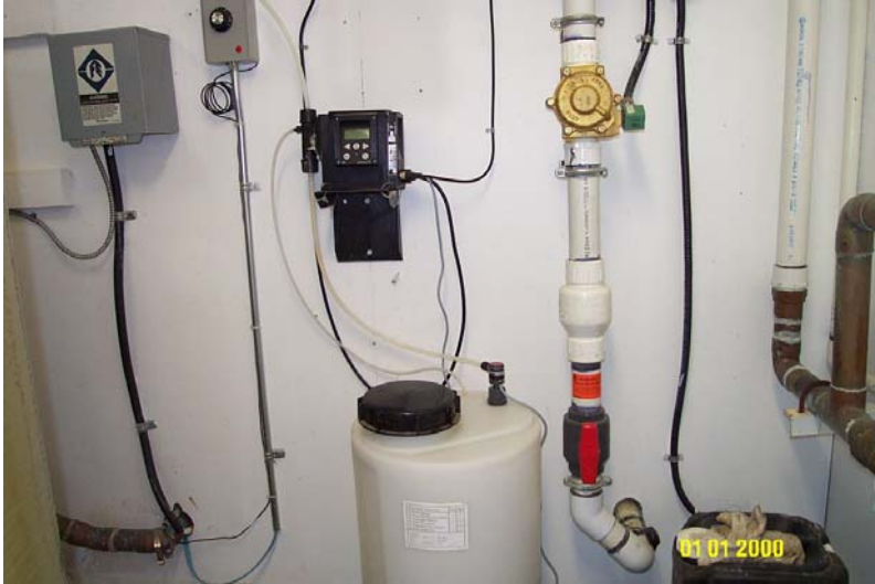
Photo 0069: 1953 Grundfos DME Chlorinator
