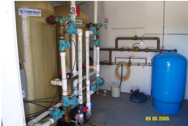
Photo 0068: 1953 Water Supply System, Pressure Tank (left), Iron Removal Tanks (right)
