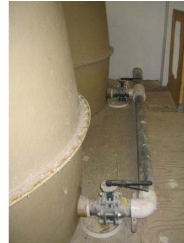
Photo 0022: 1955 Storage Tank Piping
