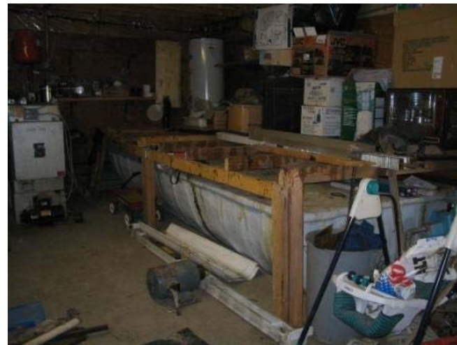
Photo 0006: YWP-D Water Storage Tank
