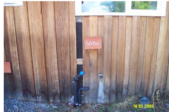
Photo 0184: YWP-B Trucked Water Intake
