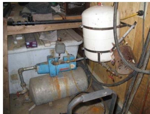
Photo 0184: YWP-D Jet Pump and Pressure Tank
