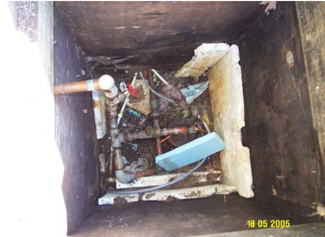
Photo 0173: YWP-A Well Head
