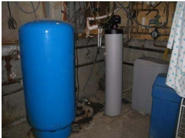
Photo 0004: YWP-A Pressure Tank (left) and Water Softener (right)
