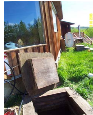
Photo 0178: YWP-A Well Head Enclosure (front), Main Office (left) and Above ground Fuel Storage Tank (right)
