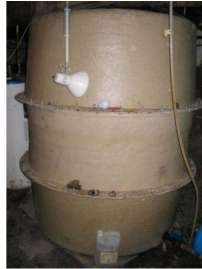
Photo 0006: YWP-B Trucked Water Storage Tank
