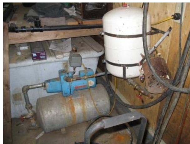
Photo 0184: YWP-D Jet Pump and Pressure Tank
