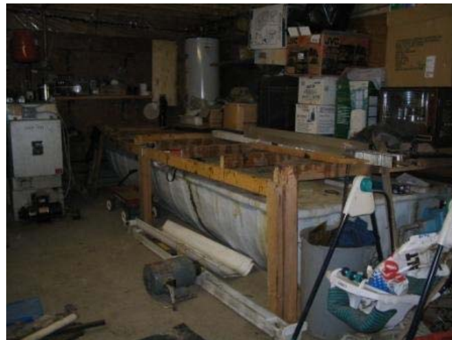
Photo 0006: YWP-D Water Storage Tank
