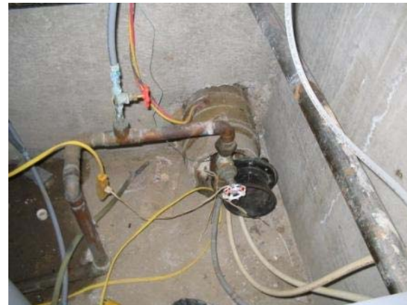
Photo 0001: YWP-A Piping in Building from Wellhead
