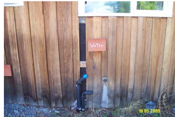
Photo 0184: YWP-B Trucked Water Intake
