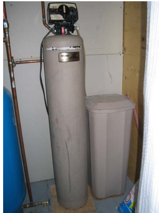
Photo 0012: M0064 Water Softener
