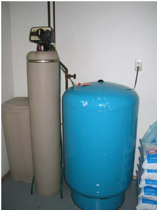
Photo 0011: M0094 Water Softener (left) and Pressure Tank (right)
