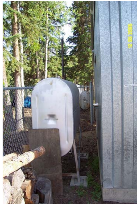
Photo 0147: M0064 and M0094 Above Ground Heating Fuel Storage Tank
