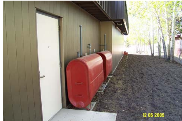
Photo 0146: M0093 Two Above Ground Storage Tanks
