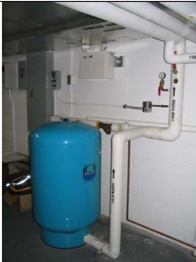
Photo 0008: M0093 Pressure Tank
