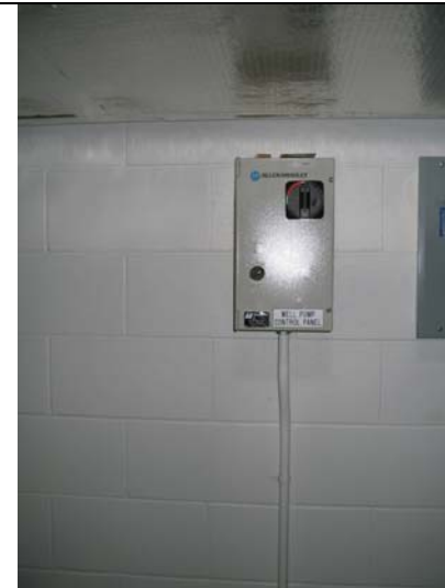
Photo 0010: M0093 Pump Control Panel
