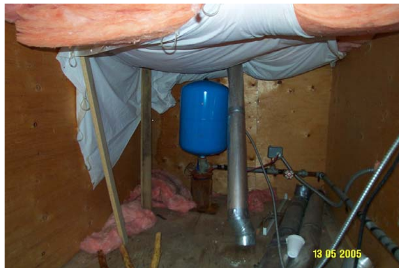
Photo 0167: M0201 Wellhead and Pressure Tank
