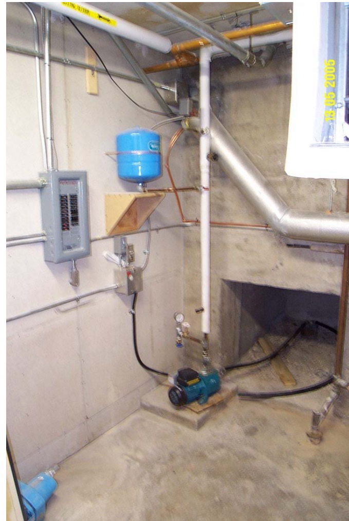
Photo 0161: 6511-A Jet Pump and Pressure Tank
