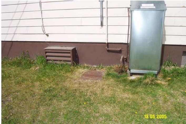
Photo 0162: 6511-A Main School Wellhead (underneath panel at center) and Above Ground Fuel Storage Tank (right)
