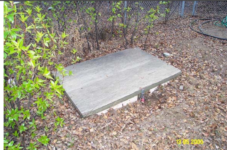
Photo 0158: 6511-C Irrigation Well Wellhead
