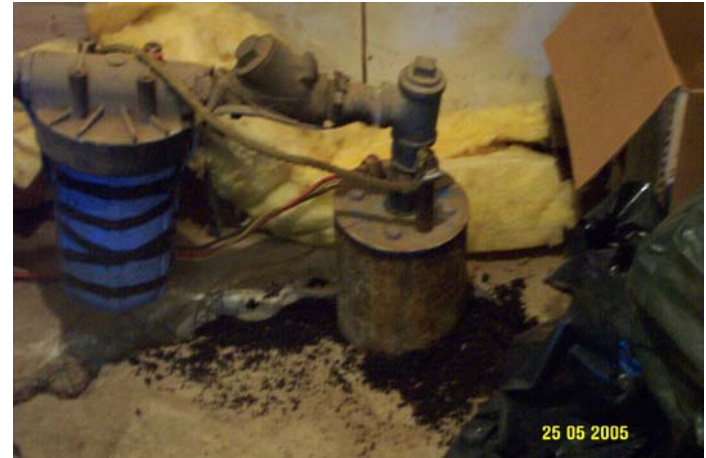
Photo 0197: 6512 Wellhead (center) and Filter (left)
