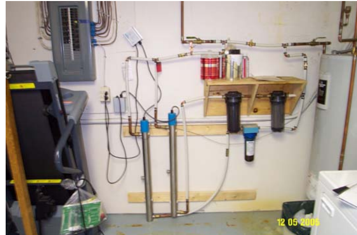
Photo 0143: 6975 Nursing Residence Water Treatment System
