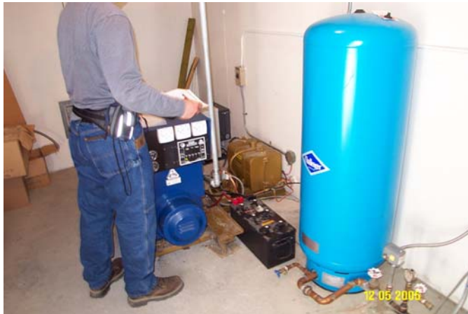
Photo 0141: 6975 Pressure Tank (right) and Backup Electrical Generator
