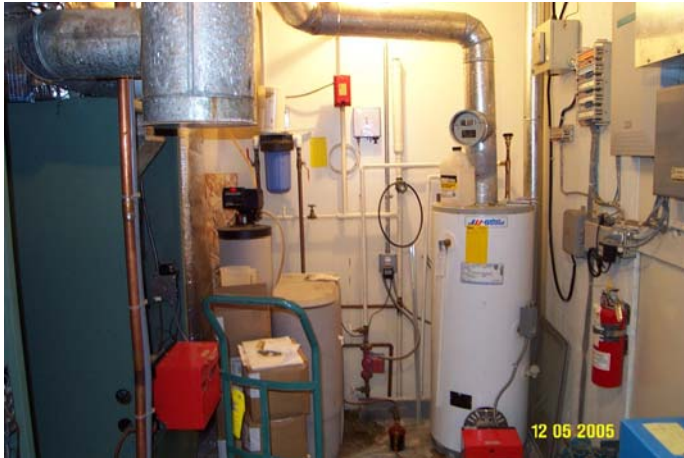
Photo 0142: 6975 Health Center Water Treatment System
