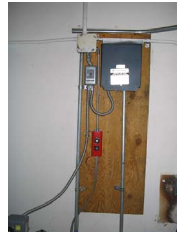
Photo 0001: 6975 Pump Control Box
