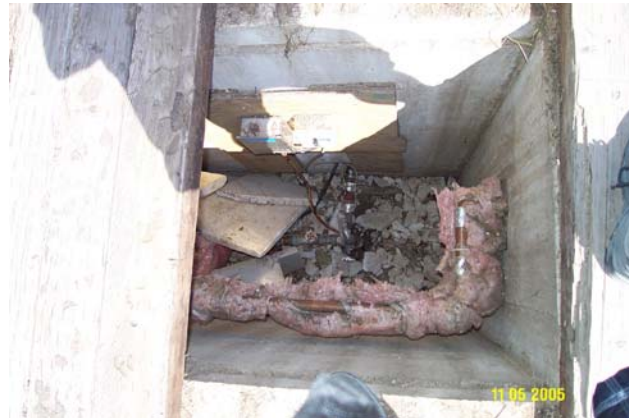
Photo 0121: 1134 Well 1 Well Head in Pit
