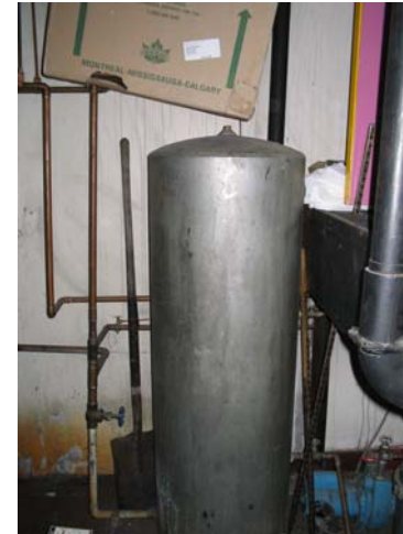
Photo 0498: 1134 Potable Water Pressure Tank
