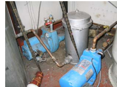
Photo 0495: 1134 Jet Pumps and Tank
