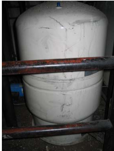
Photo 0497: 1134 Heating Expansion Tank
