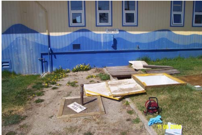
Photo 0115: 1134 Wells 1 and 2, Water Fill, Underground Fuel Storage Tank
