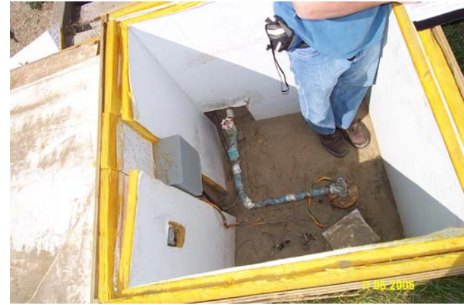
Photo 0120: 1134 Well 2 Well Head in Pit
