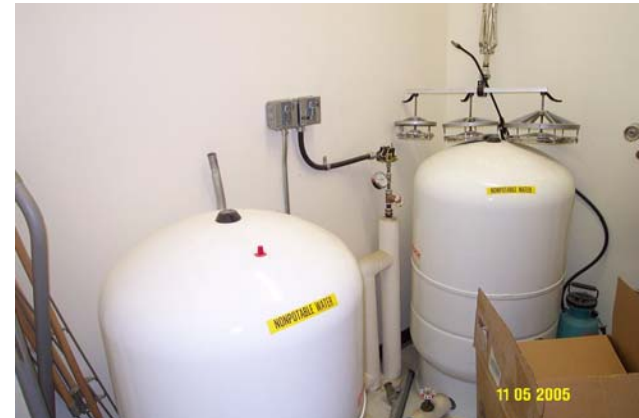
Photo 122: 1134 Pressure Tanks and Flow Switch
