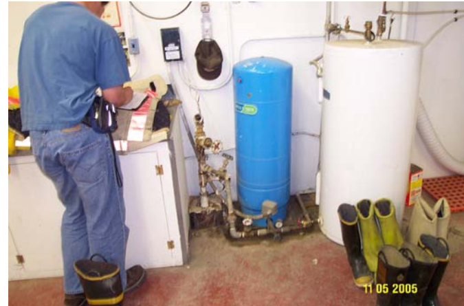
Photo 0129: 1137 Well, Pressure Tank and Pump Controls
