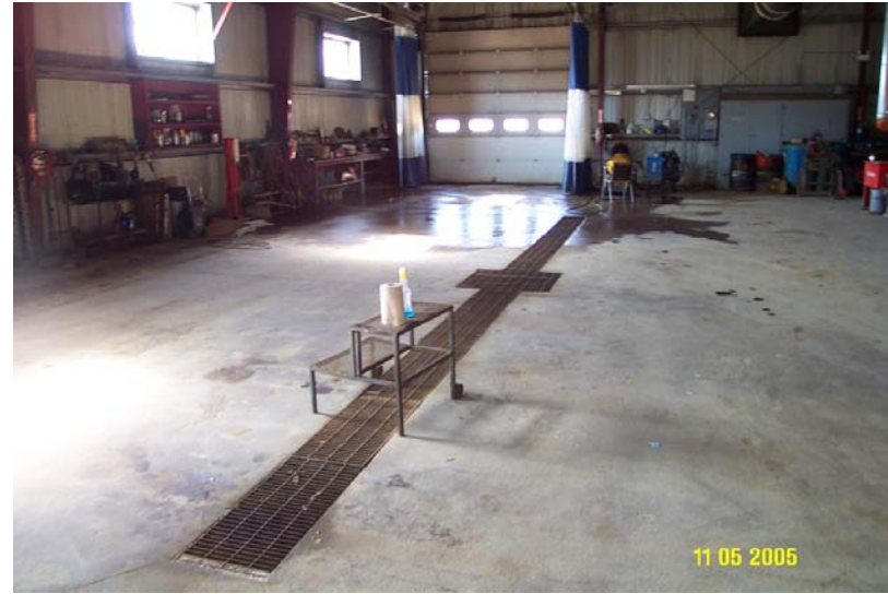
Photo 0134: Floor Drain System
