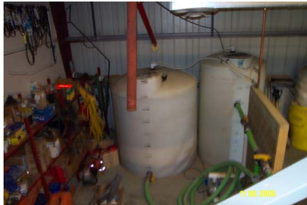
Photo 0135: Water Tanks/Brine Tanks
