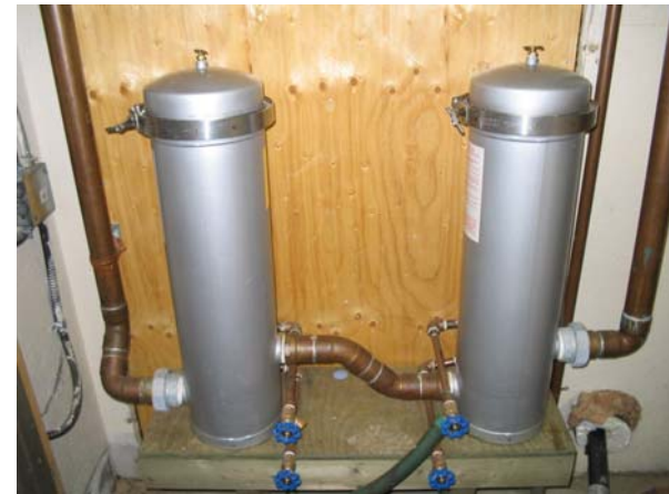
Photo 0486: 1500 Filter System, 1 Micron Filter (left) and 10 Micron Filter (right)
