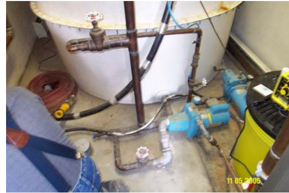
Photo 0109: 1500 Jet Pump and Backup Water Reservoir
