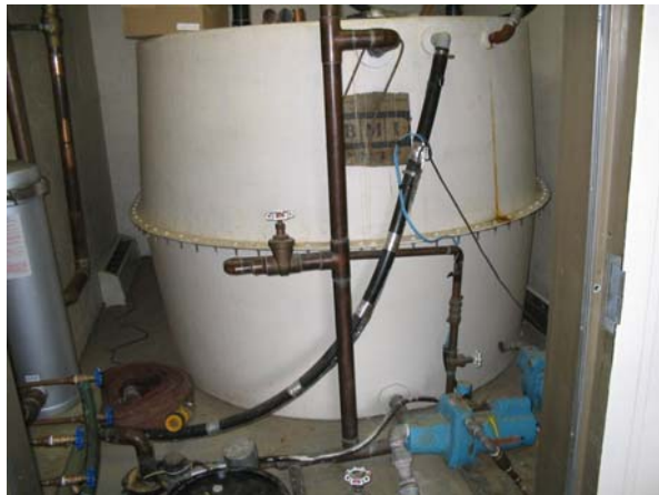
Photo 0484: 1500 Water Storage Tanks
