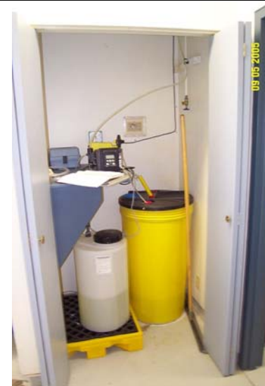
Photo 0072: 1334 DME Chlorinator and LMI Chlorinator back-up system.
