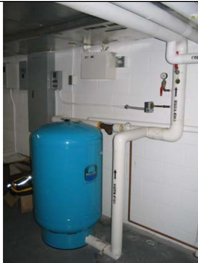
Photo 0008: M0093 Pressure Tank
