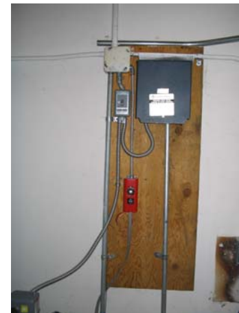
Photo 0001: 6975 Pump Control Box
