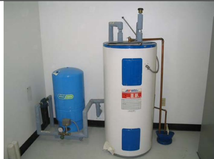
Photo 0018: 6522 Pressure Tank (left) and Water Heater (right)
