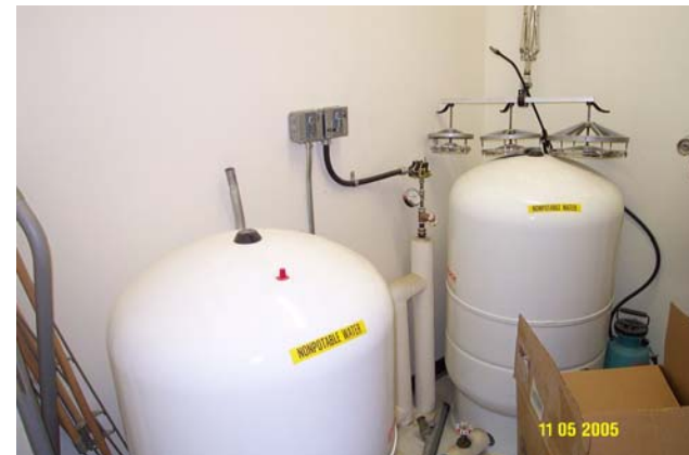
Photo 122: 1134 Pressure Tanks and Flow Switch
