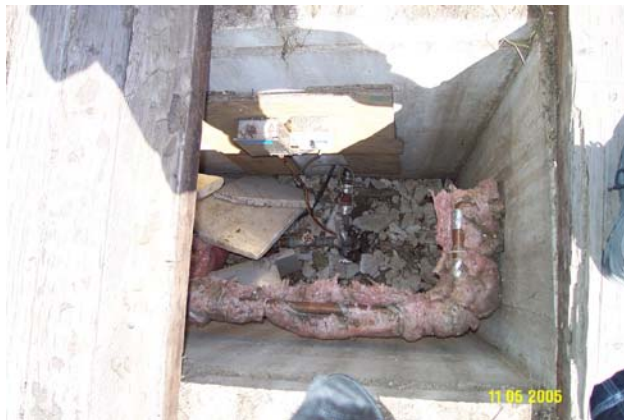
Photo 0121: 1134 Well 1 Well Head in Pit
