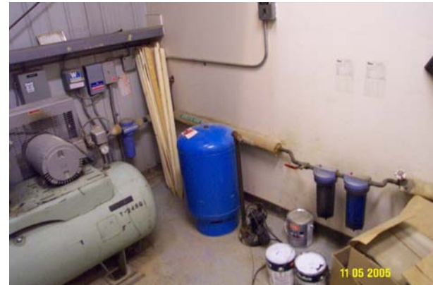
Photo 0136: Pressure Tank and Three In-Line Filters
