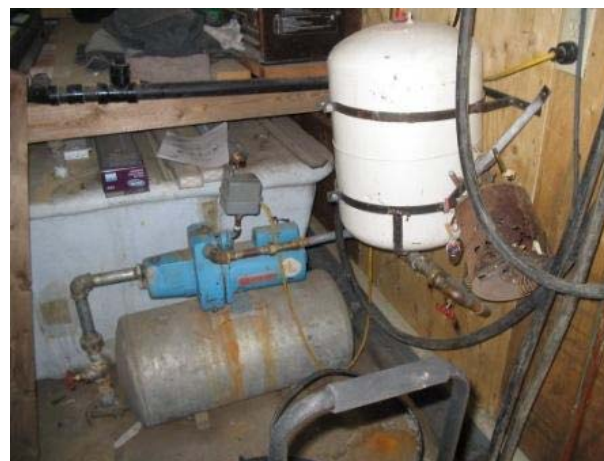
Photo 0184: YWP-D Jet Pump and Pressure Tank
