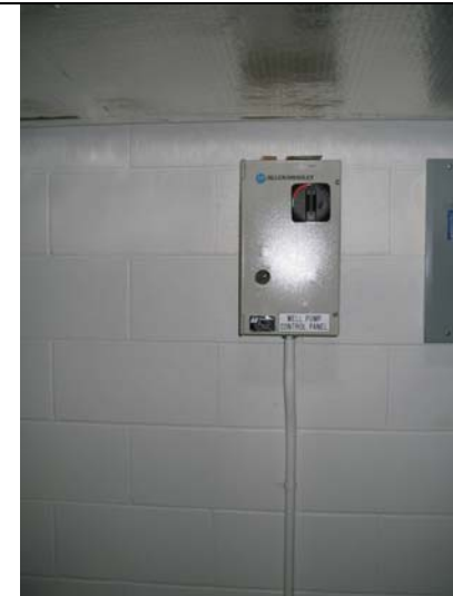
Photo 0010: M0093 Pump Control Panel
