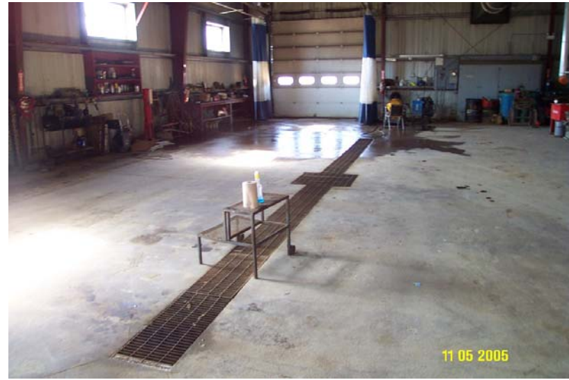
Photo 0134: Floor Drain System
