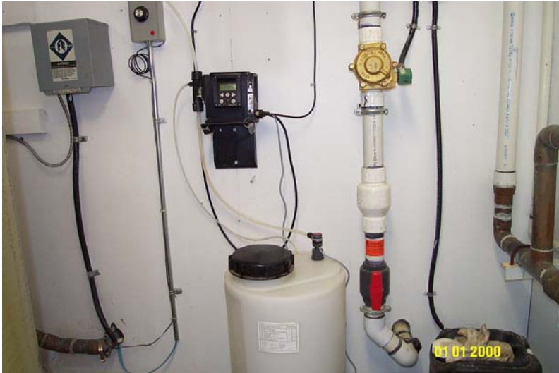
Photo 0069: 1953 Grundfos DME Chlorinator
