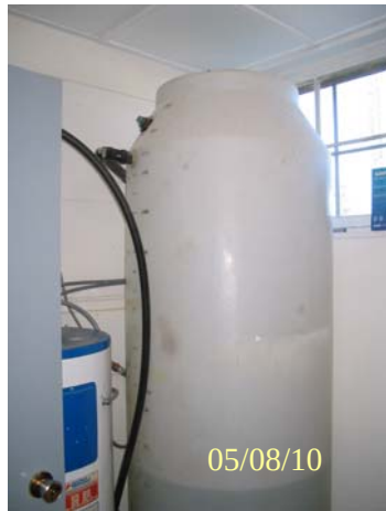
Photo 141: 1131 Water storage tank.
