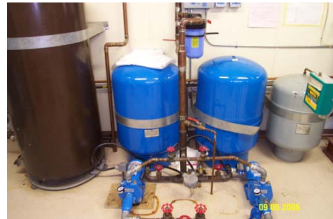
Photo 0086: 1322 Pressure Tanks and Filter
