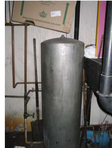
Photo 0498: 1134 Potable Water Pressure Tank
