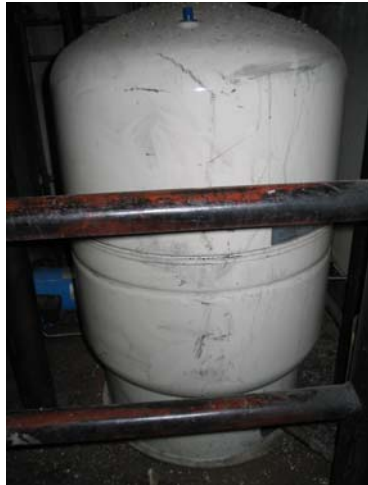
Photo 0497: 1134 Heating Expansion Tank
