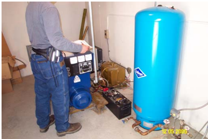
Photo 0141: 6975 Pressure Tank (right) and Backup Electrical Generator
