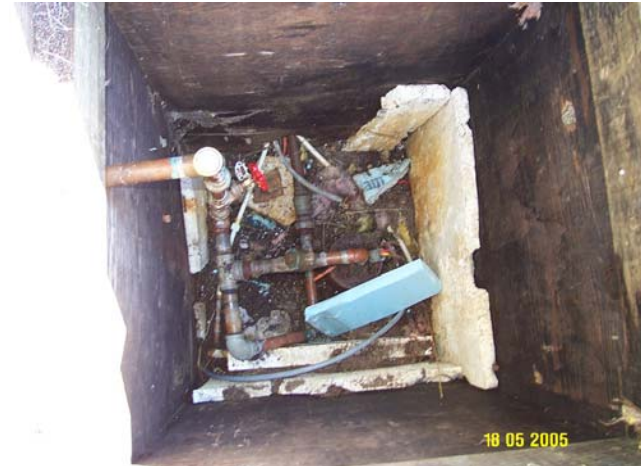
Photo 0173: YWP-A Well Head
