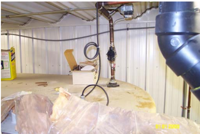
Photo 0107: 1950 Solenoid and Water Storage Tank
