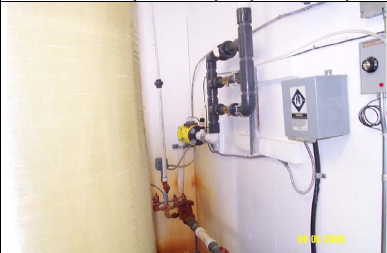
Photo 0070: 1953 Pumphouse Iron Duplex Injection Chlorine System
