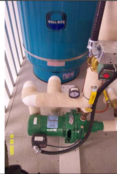
Photo 0098: 1421 Pressure Tank and System
