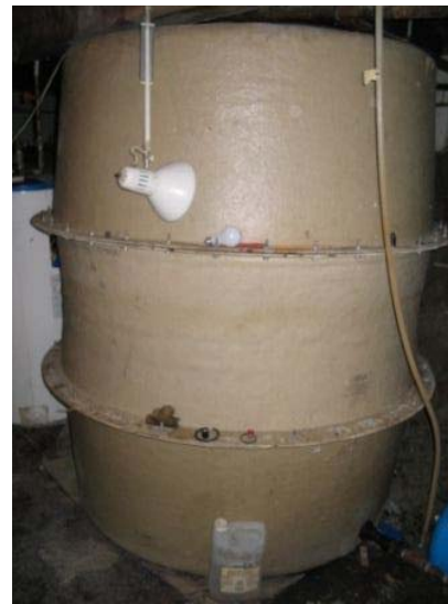
Photo 0006: YWP-B Trucked Water Storage Tank
