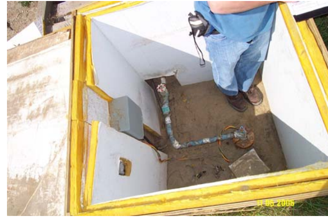
Photo 0120: 1134 Well 2 Well Head in Pit
