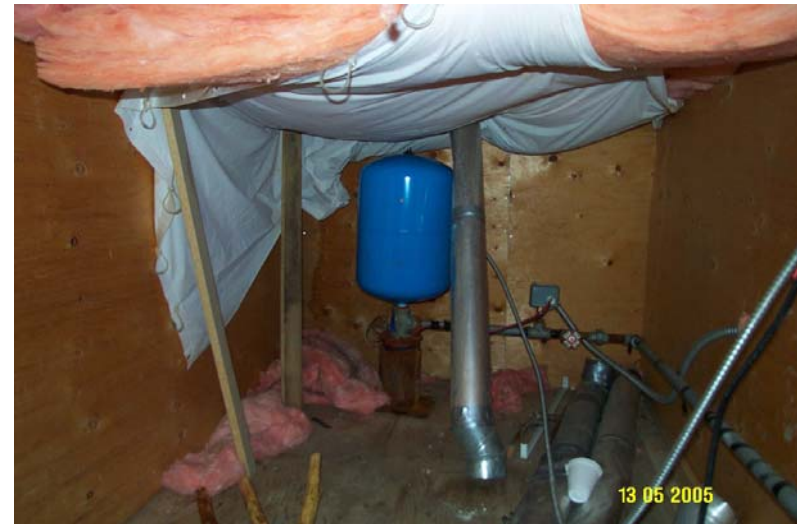
Photo 0167: M0201 Wellhead and Pressure Tank
