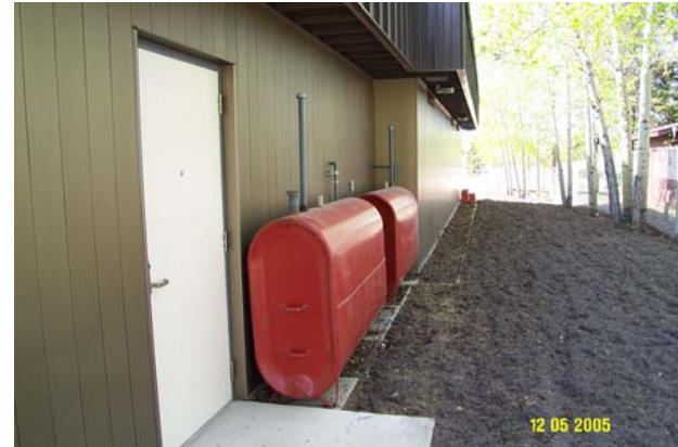
Photo 0146: M0093 Two Above Ground Storage Tanks
