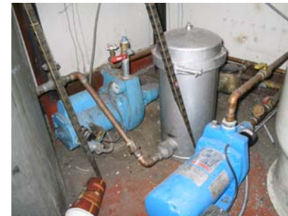
Photo 0495: 1134 Jet Pumps and Tank
