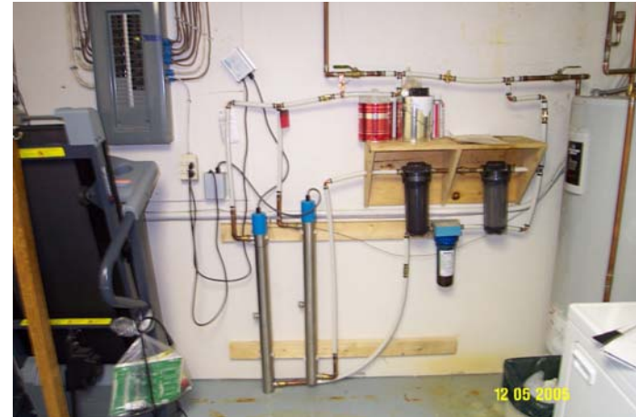
Photo 0143: 6975 Nursing Residence Water Treatment System
