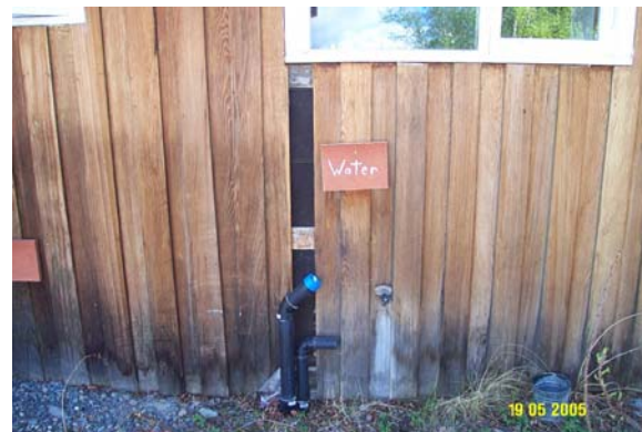
Photo 0184: YWP-B Trucked Water Intake
