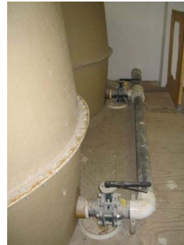
Photo 0022: 1955 Storage Tank Piping
