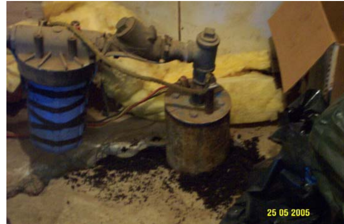
Photo 0197: 6512 Wellhead (center) and Filter (left)
