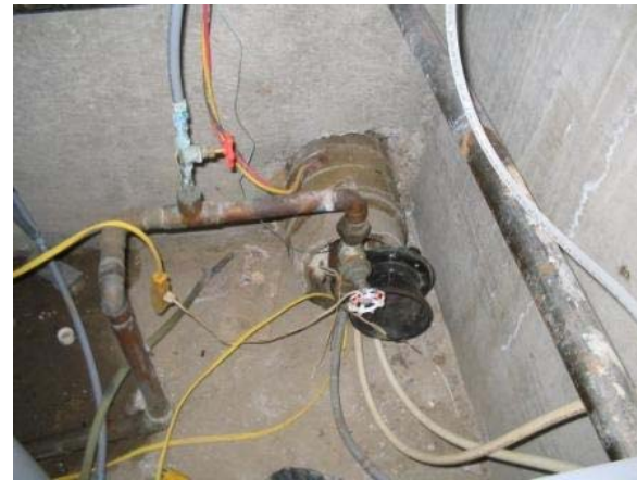
Photo 0001: YWP-A Piping in Building from Wellhead
