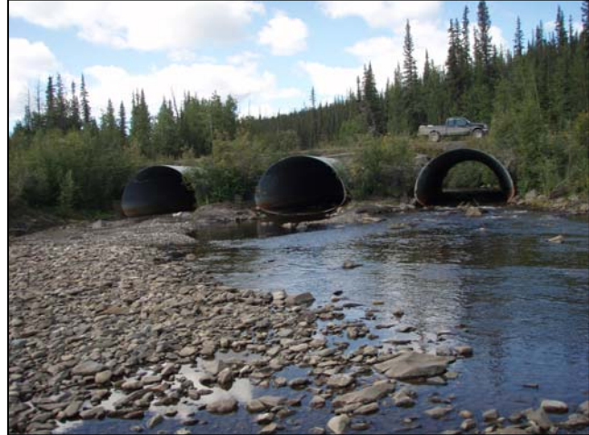
Figure 2.25: Culverts at the Davies Creek crossing of the Dempster Highway. (Photo: A. von Finster, DFO)
