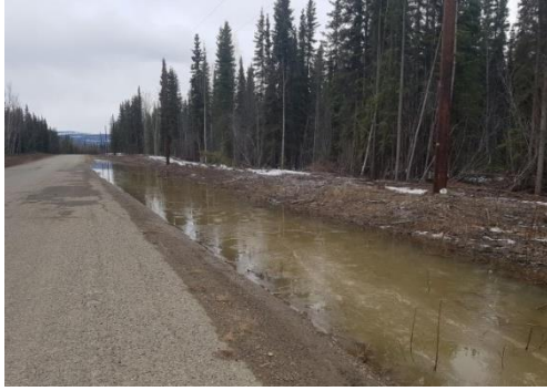
April 26 th , 2018 ditch conditions along Silver Trail
