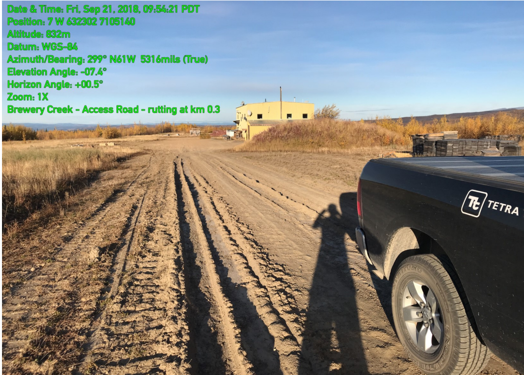
Photo 1: Rutting near camp at about km 0.3.
