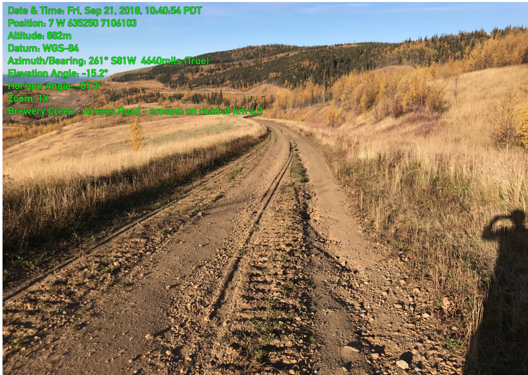
Photo 2: Minor erosion on road surface at about km 4.3.
