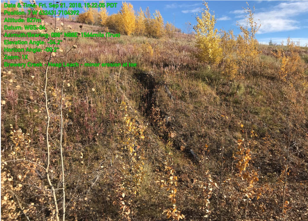
Photo 21: Minor erosion at toe of heap leach pile.
