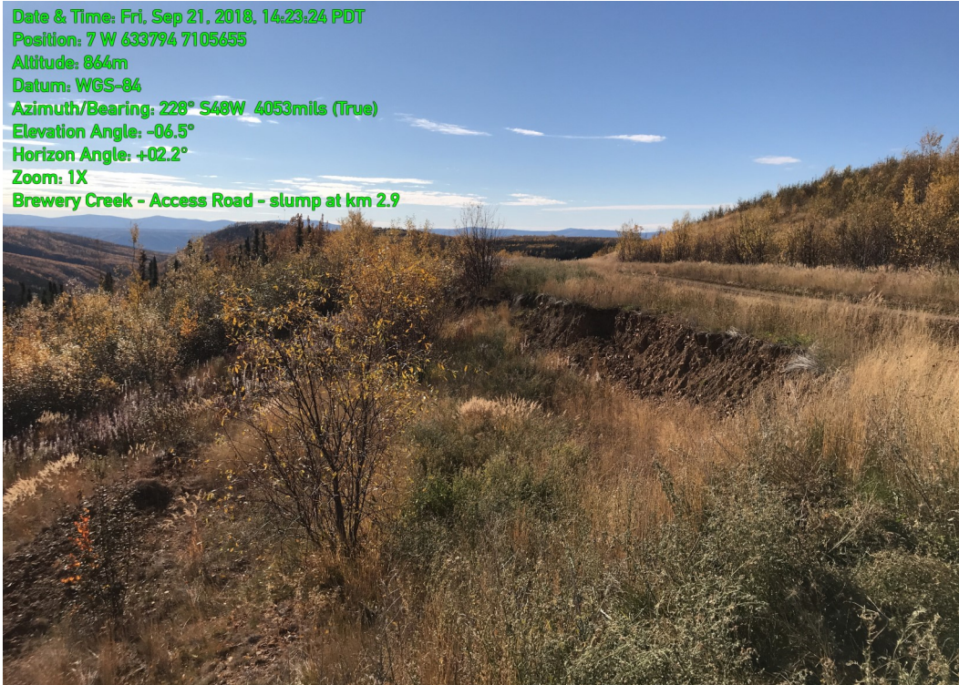
Photo 11: Slump on downhill side of road at about km 2.2 (recorded as km 2.9 in the field). Note soil exposed in approx. 1.5 m high headscarp below road, and setback of about 2 to 3 m from road
