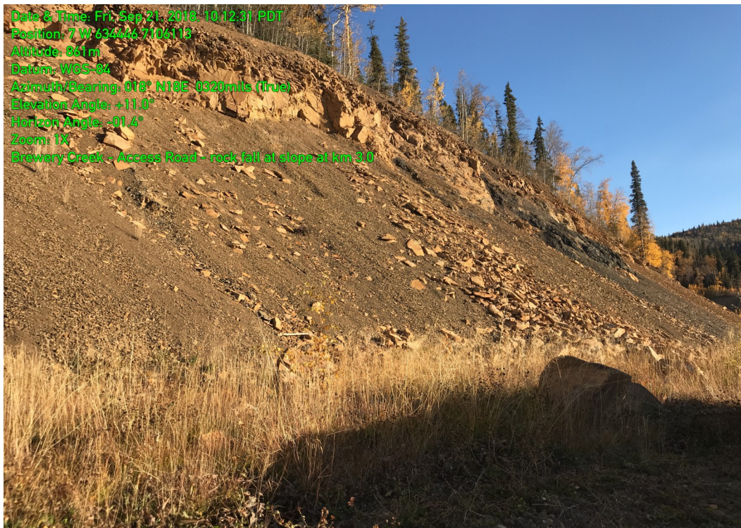
Photo 6: Recent rock fall debris on face of slope at about km 3.0. Note boulder near edge of road in bottom left of the frame (in shadow).
