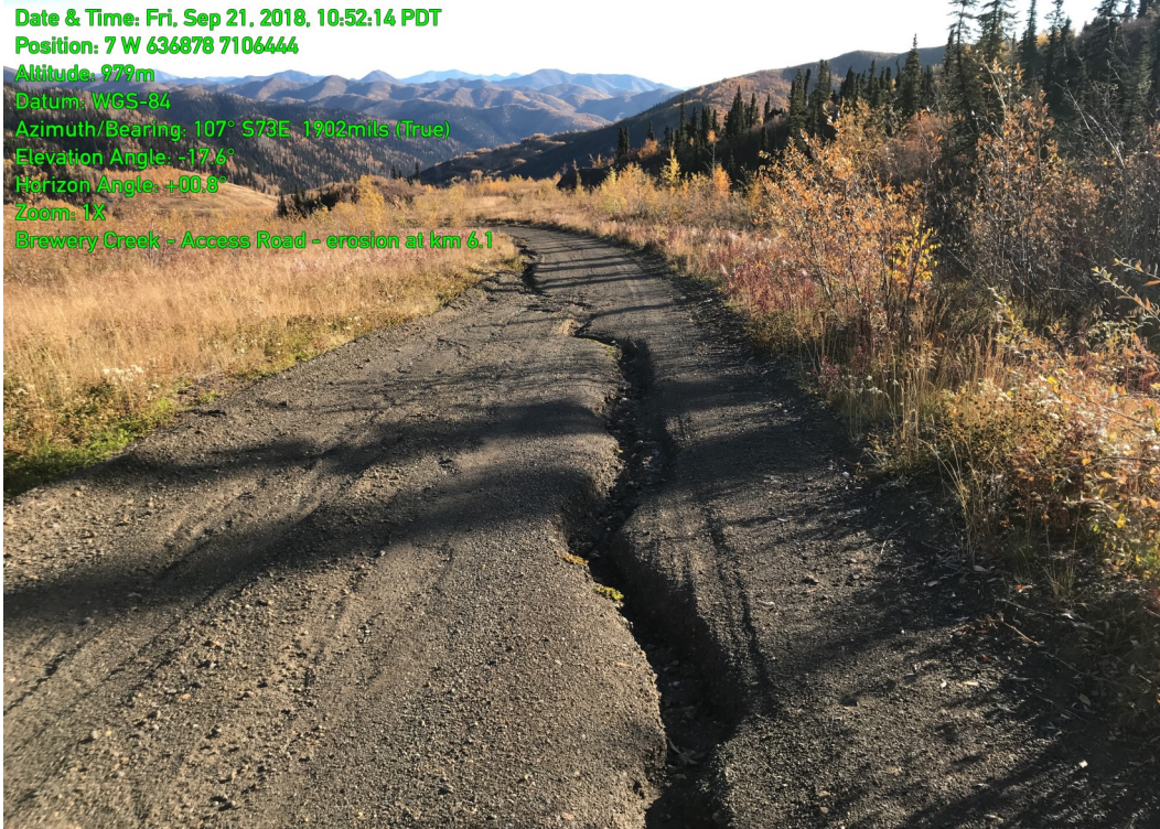
Photo 3: Erosion gully on road surface at about km 6.1.
