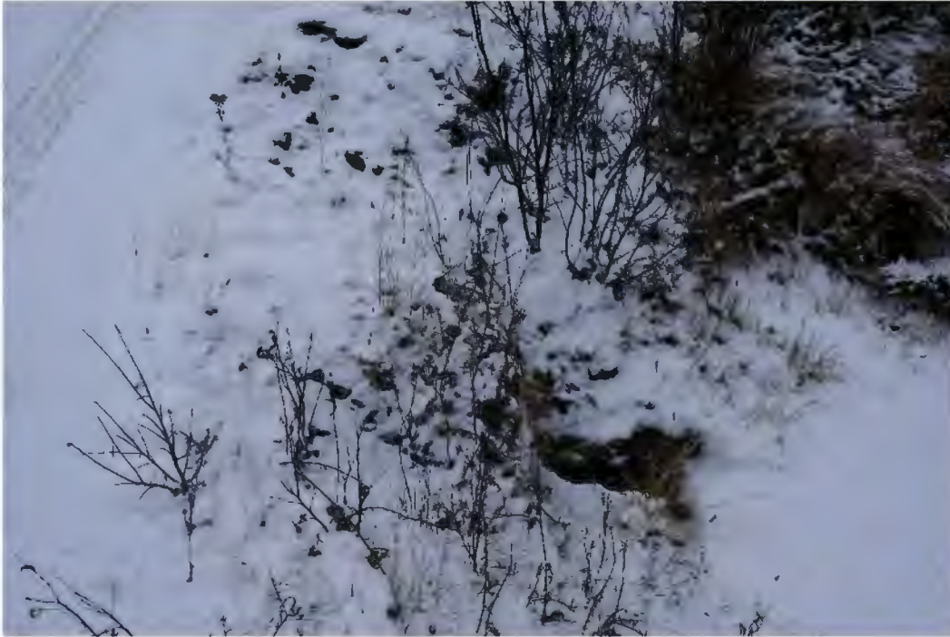
Photograph 13: Culvert Inlet beneath road at North Williams Creek
