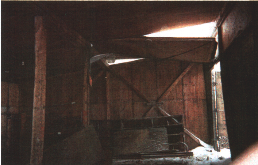
Photograph 6: Section of roof on maintenance shed that is in danger of collapse as weight of snow increases
