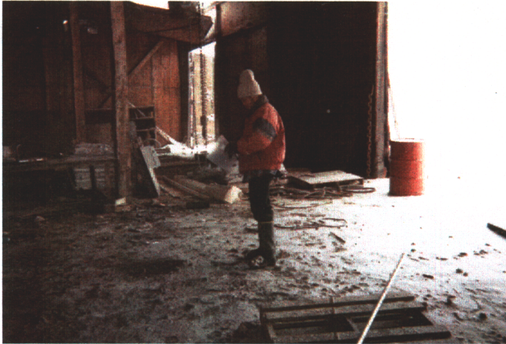
Photograph 7a,b: Stained soil in service bay of maintenance building (location of Site 1 sample)
