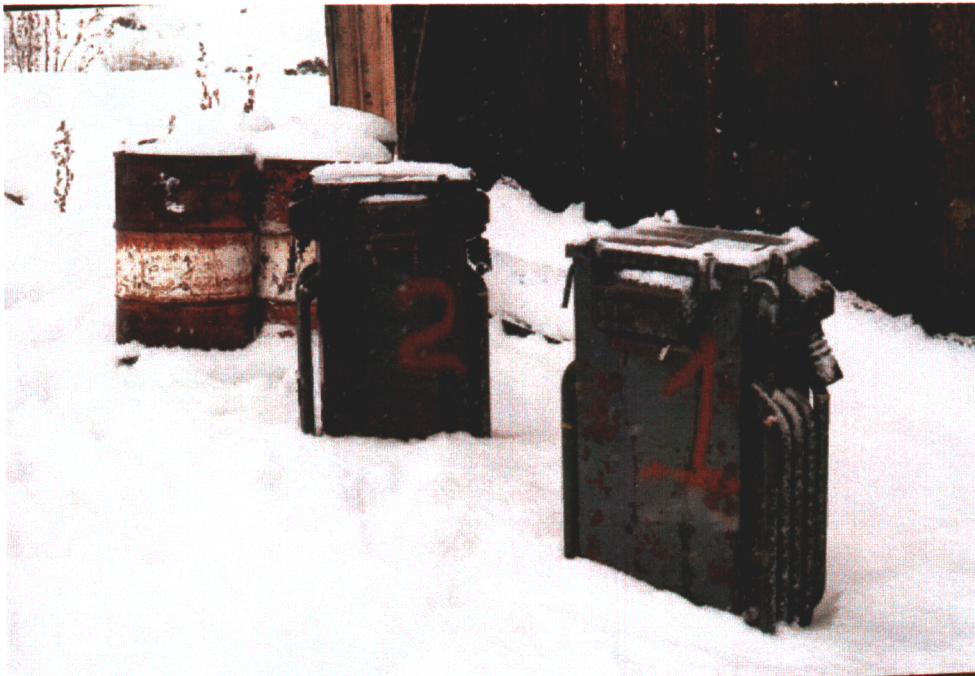
Photograph 12: Five drums located adjacent to generator section of maintenance shed – one contained gas, two contained waste oil and two were empty plus two transformers
