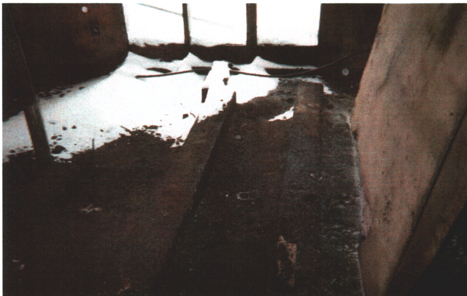
Photograph 8: Stained soil on floor of generator part of maintenance shed (Site 2 sample)
