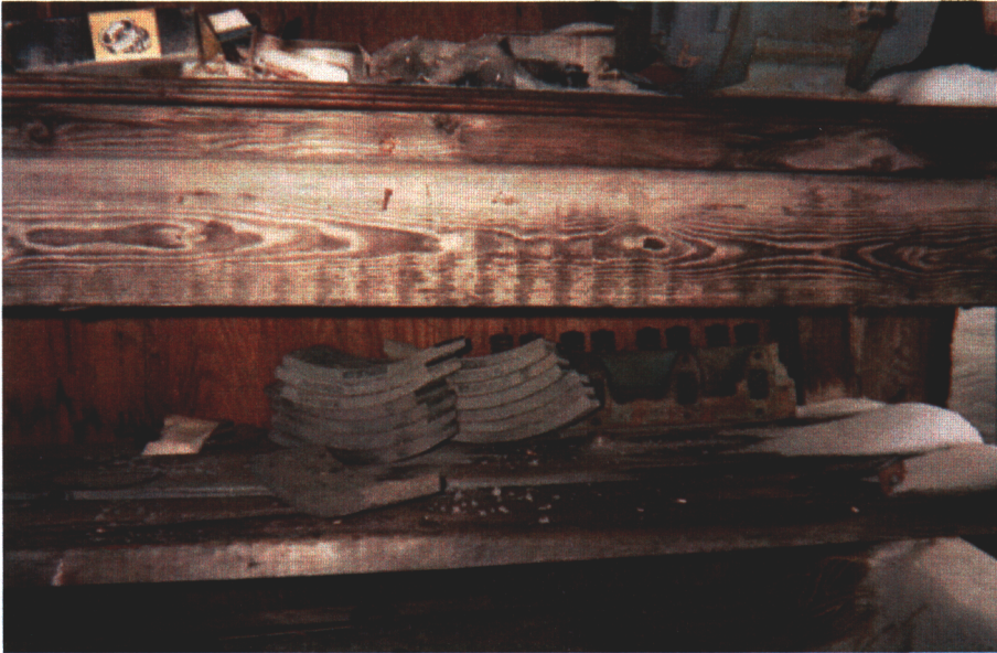
Photograph 17: Asbestos brake pads stored in maintenance building.
