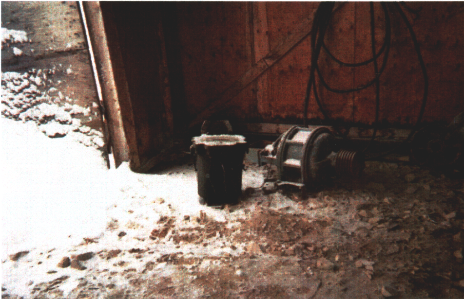
Photograph 19: Old cast iron case transformer inside maintenance shed
