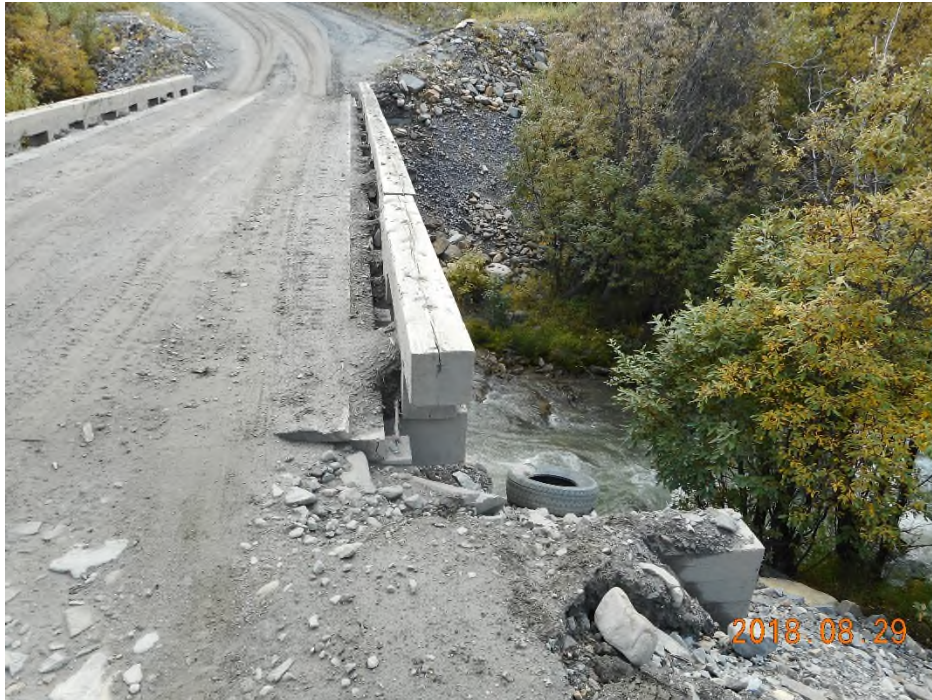
Photo 5: Bellekeno Haul Road bridge crossing Lightning Creek – erosion protection is required at the ends of the approaches to the bridge to protect the abutments and the bridge deck
