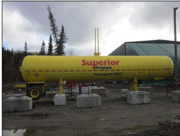
Photo 22: Propane Storage Tank
