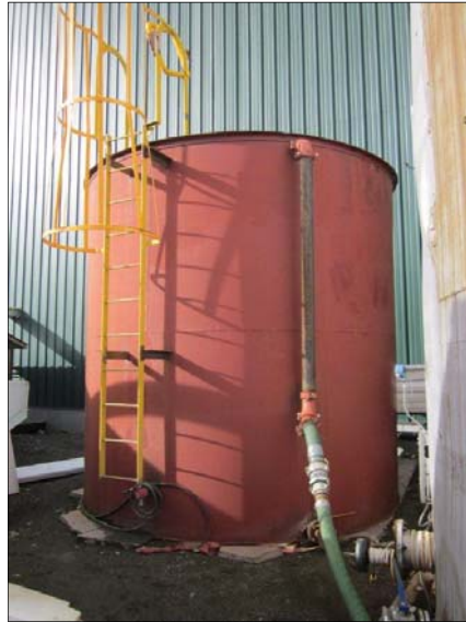
Photo 15: Fresh Water Tank
