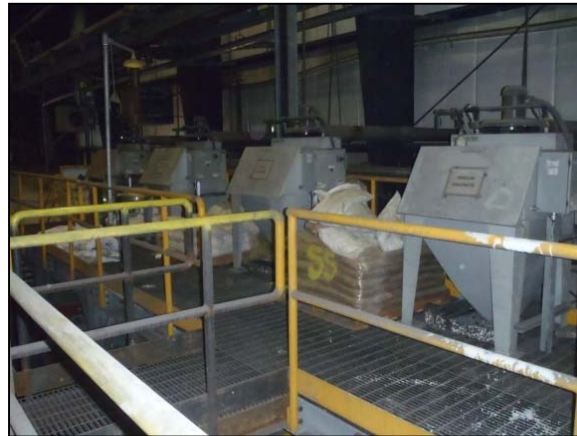
Photo 17: Reagent Mixing Station
