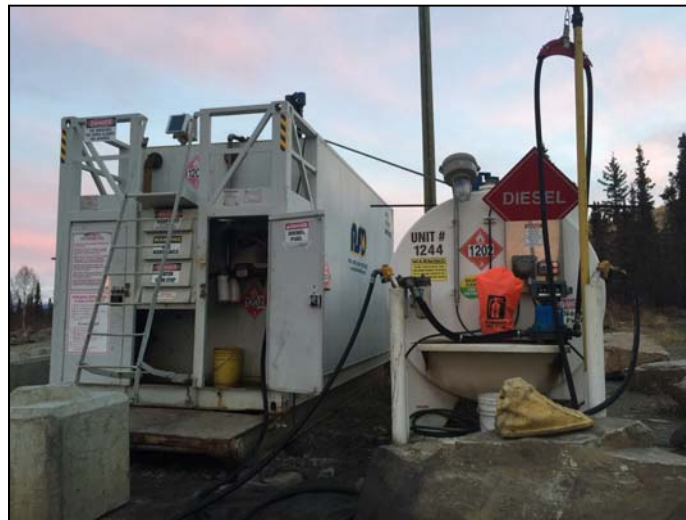
Photo 21: Diesel Storage Tanks
