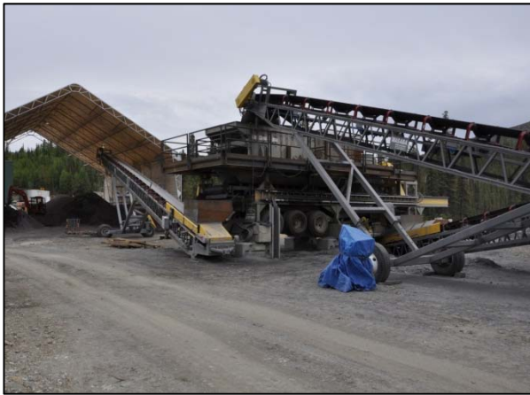
Photo 2: Primary, Secondary Crushing
