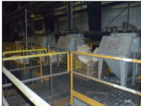
Photo 16: Reagent Mixing Station
