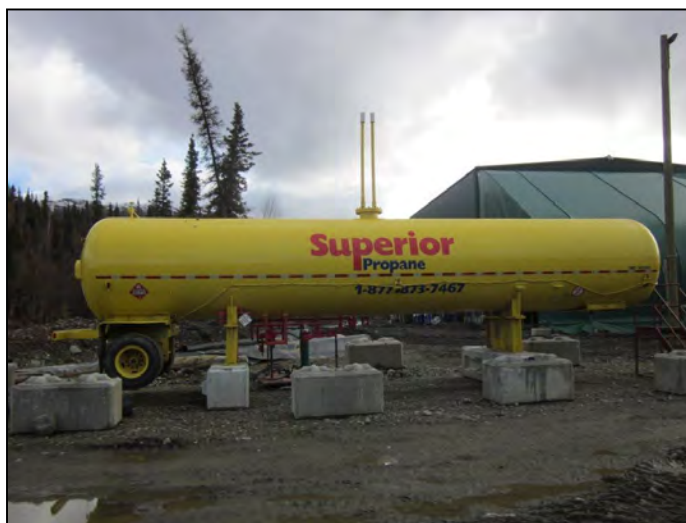
Photo 21: Propane Storage Tank
