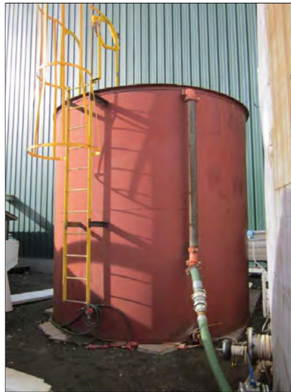
Photo 14: Fresh Water Tank
