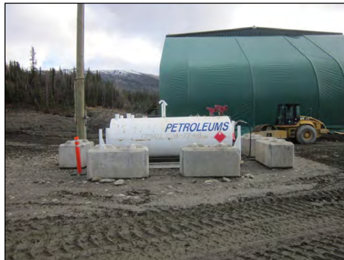
Photo 20: Diesel Storage Tanks
