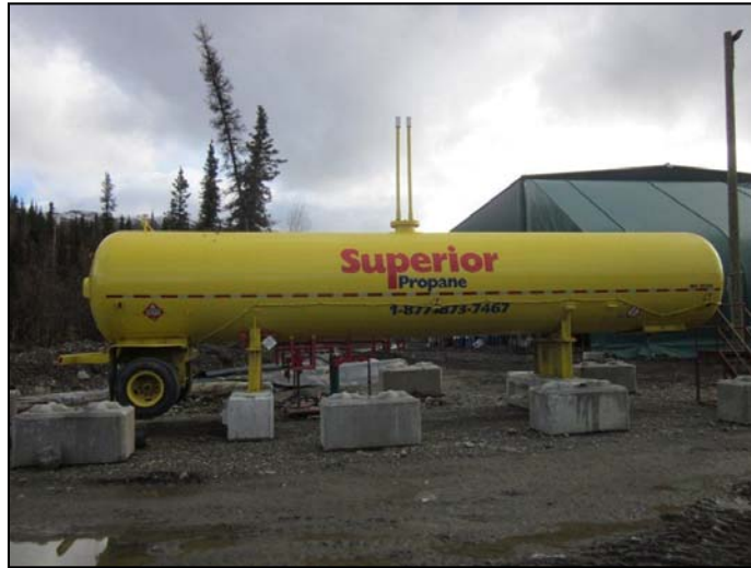
Photo 22: Propane Storage Tank
