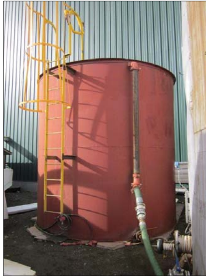
Photo 15: Fresh Water Tank
