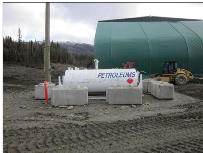
Photo 21: Diesel Storage Tanks
