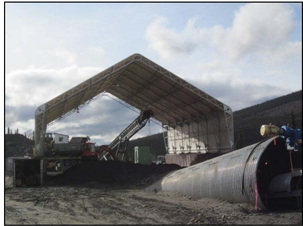
Photo 3: Fine Ore Storage
