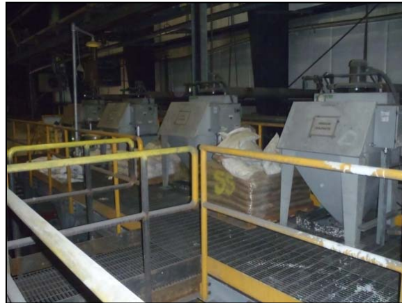
Photo 17: Reagent Mixing Station
