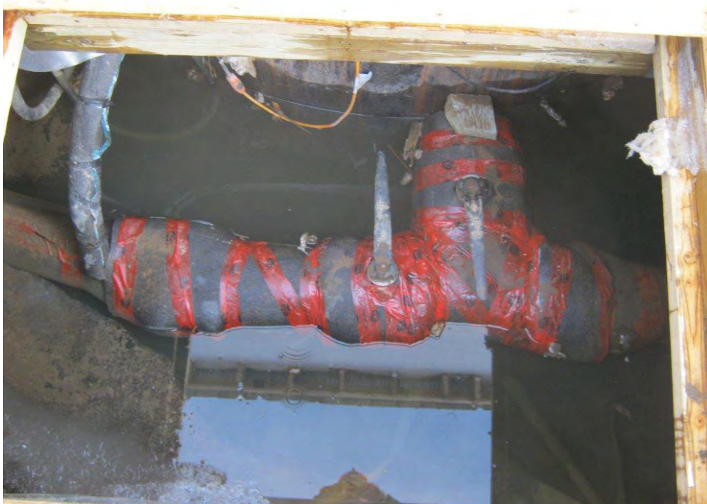
Figure 8 - Bioreactor Discharge Valves
